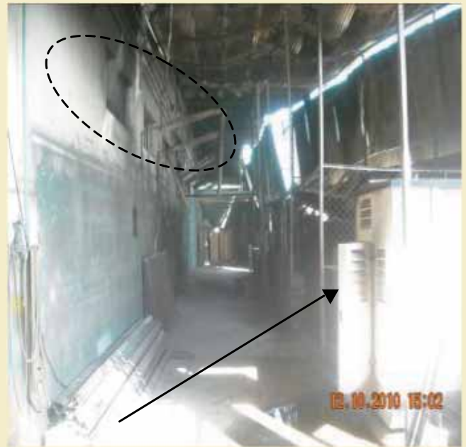
Location of the DG set and the Ventilators
