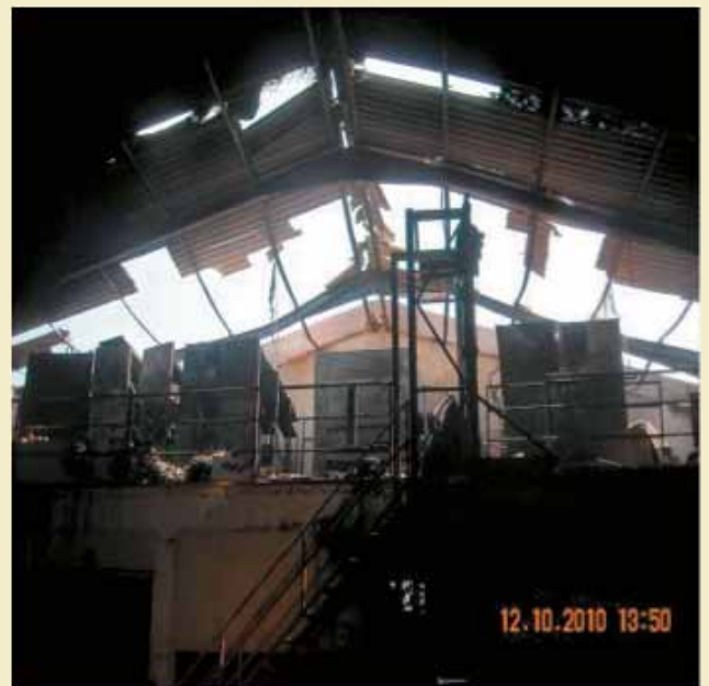
Damaged roof above the mezzanine floor
