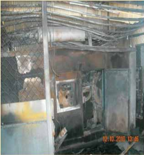
The DG set where the fire is first noticed
